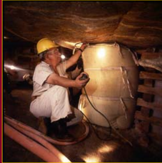
“Pack in the pipe”
